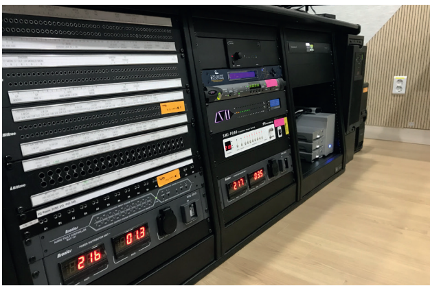
The REF 10 and iClock installed in Mixing Studio 2
